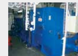
Synchronous generators, Diesel Electric propulsion
