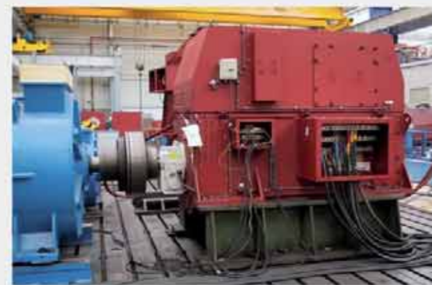
2 off main generators
