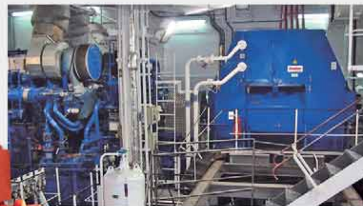
Synchronous generators, for electric needs
