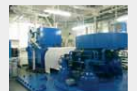
Asynchronous motors, Diesel Electric propulsion
